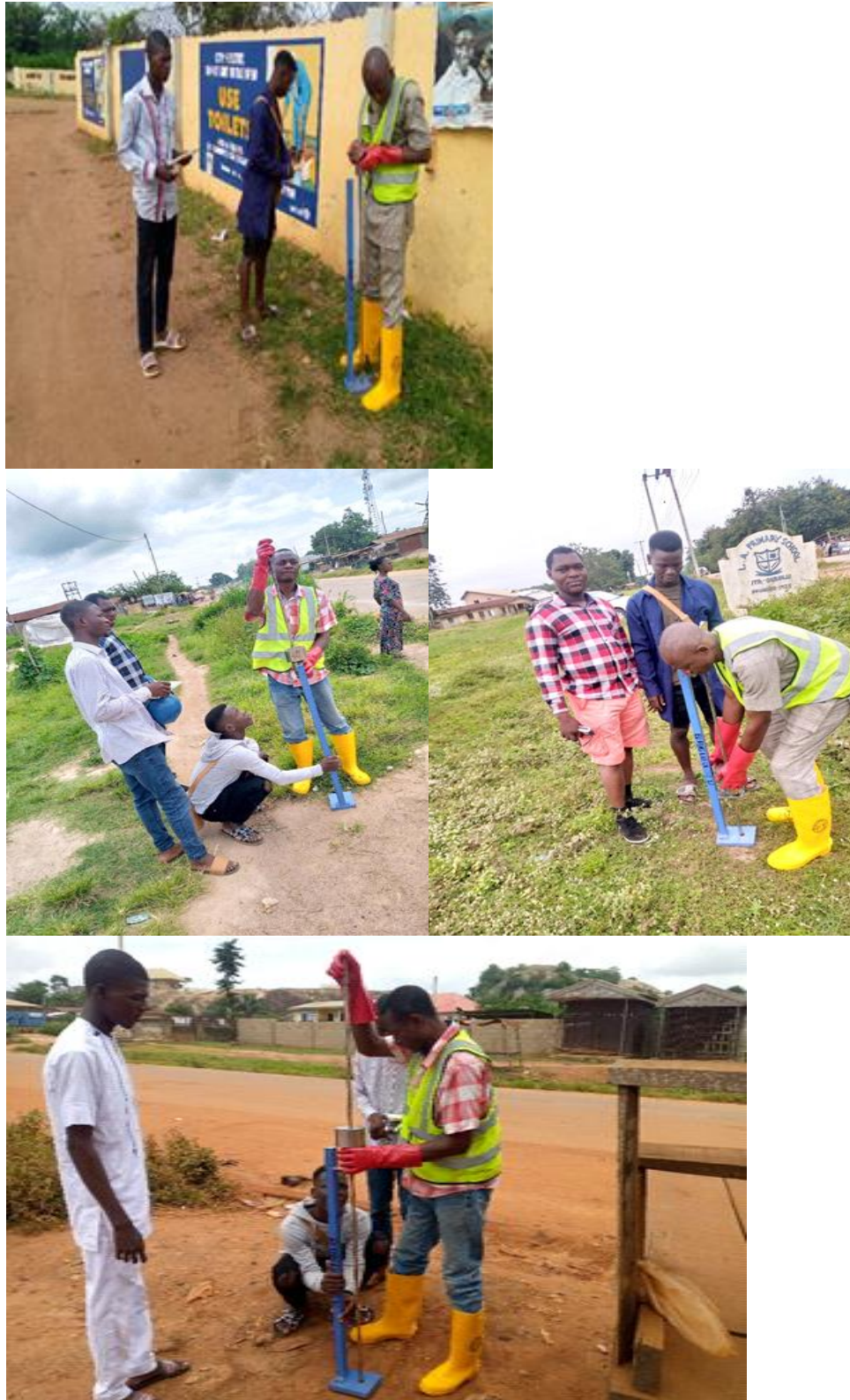
Fig. 6 DCPT Field Survey carried out along Akure – Ado Ekiti Highway at different locations
